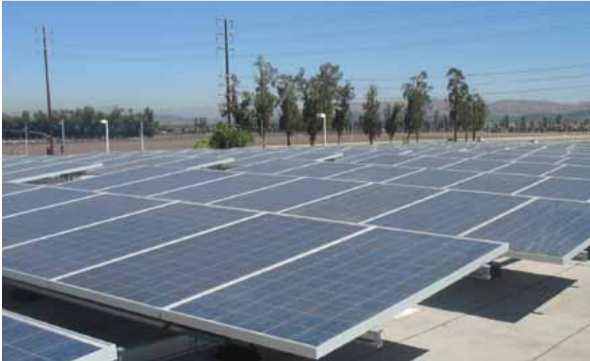
Rooftop solar installation on the District's Maintenance and Operations Facility. Photo: Joe Hoffman, IUSD's Director of Maintenance and Operations
