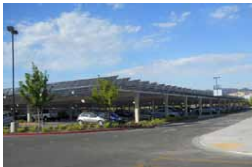
102 kW solar PV system at Dougherty Valley High in San Ramon, CA.
