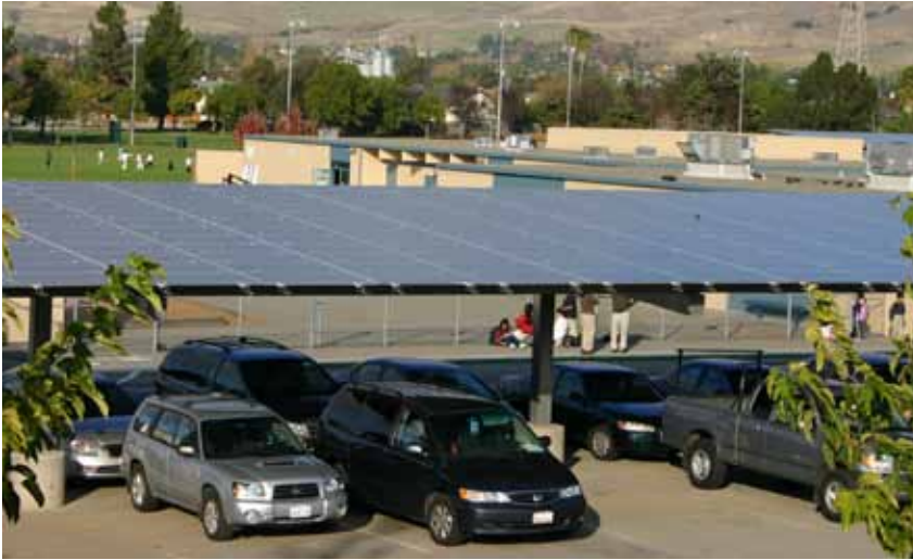
Curtner Elementary School in Milpitas benefits from a 139 kW carport solar system. Photo: Chevron Energy Solutions
