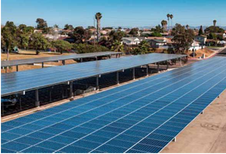
Nearly completed 507 kW carport solar power system at Montgomery High School in San Diego.
